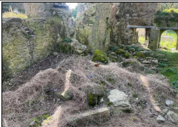
Plate 12: View of building rubble from NE.
